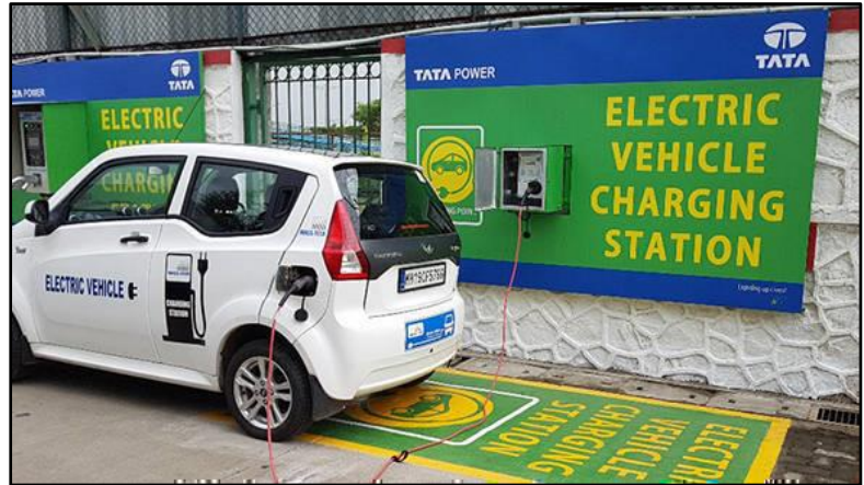
Figure 2: EVs Charging Station by TATA POWER
